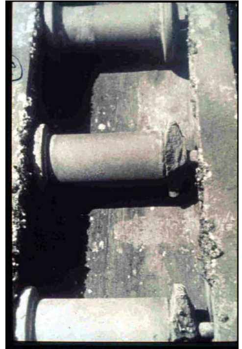
BROKEN ROLLER FLANGES
