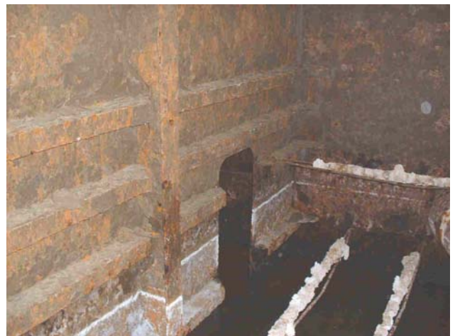
HEAVY RUST SCALE
