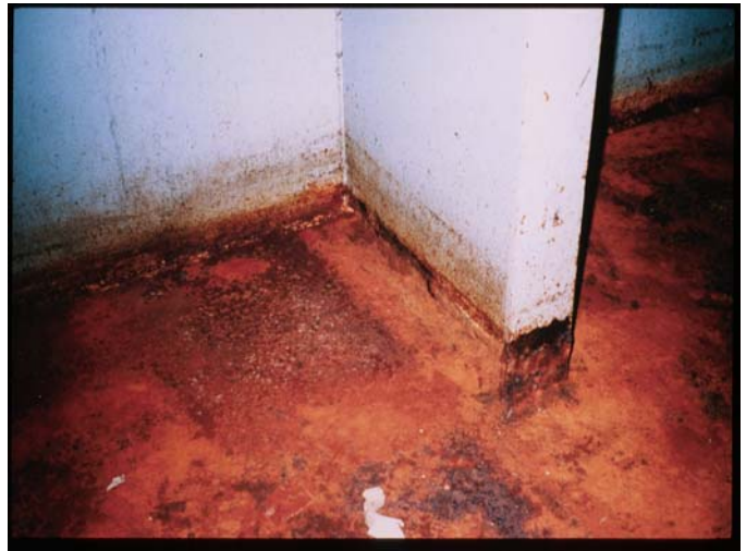
RUST SCALE AT SAFETY DECK
