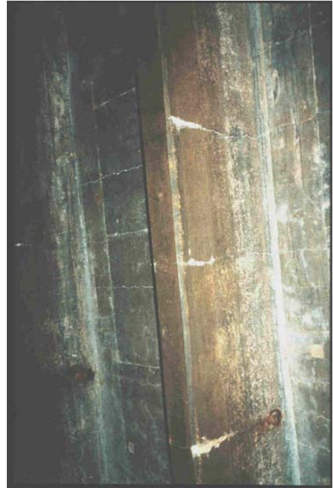
1 st STAGE - GRACKS
