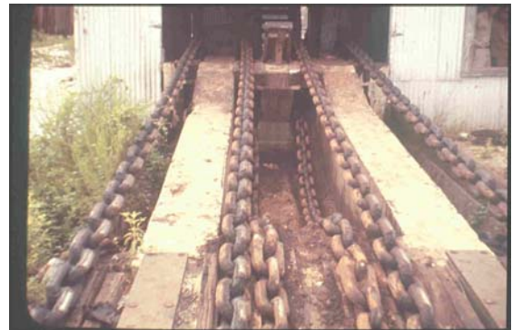
CHAIN TOO LOOSE
