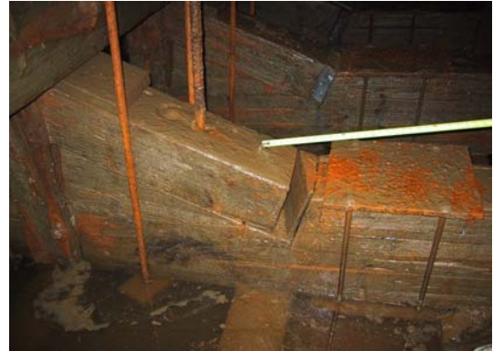
GAP IN TIMBER TRUSS
